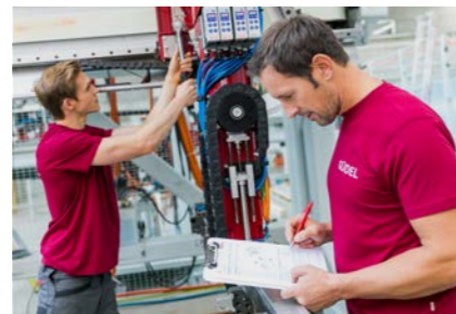
Competently maintaining systems
